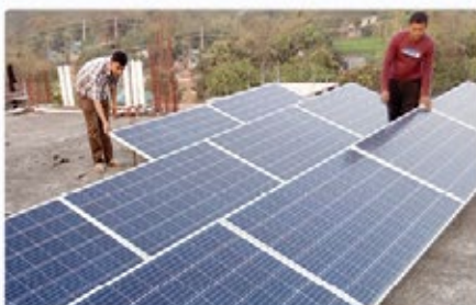
New solar panels keep security lights and CCTV cameras operating 24 hours a day
