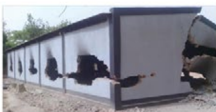
This church building in Loropeni was all but demolished in the three-day attack
