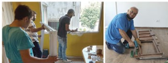
Many damaged homes were left without windows or secure doors. Barnabas supported urgent basic repairs to make houses safe and secure for families
